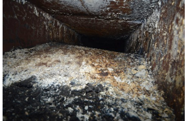
Fig 2. Oil and fat deposits that have been fire-affected.
